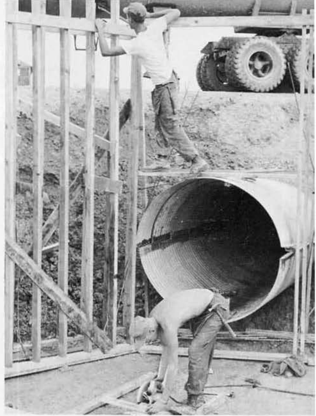
Large culvert for the Marines is supplied by BUL3 Dan Eppinga, Clarendon Hills, Ill. (top) and BURCN Don MacLean, Ithaca, N.Y.; both Charlie Co. Seabees.
