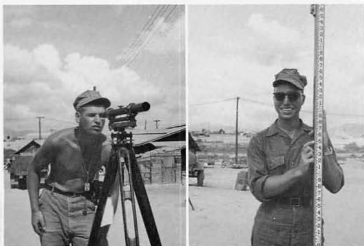
EADCN Griggs and EASCN Welter survey for road improvements in the camp area.
