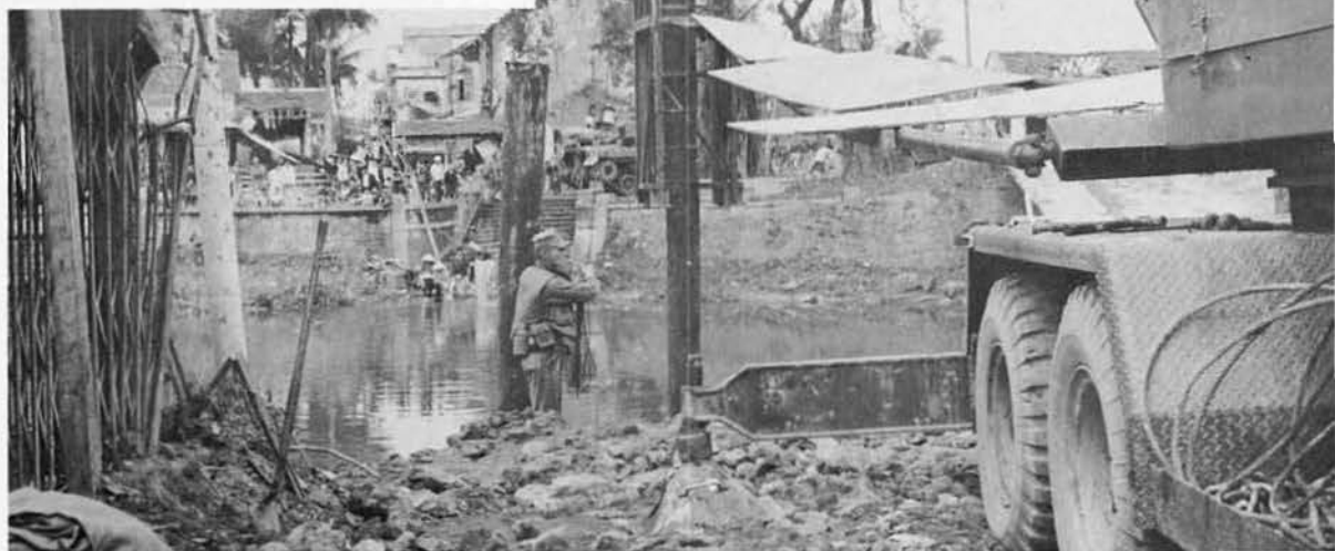
Alpha Company equipment operators and Delta Company builders team up to set pilings for a bridge in Hue.
