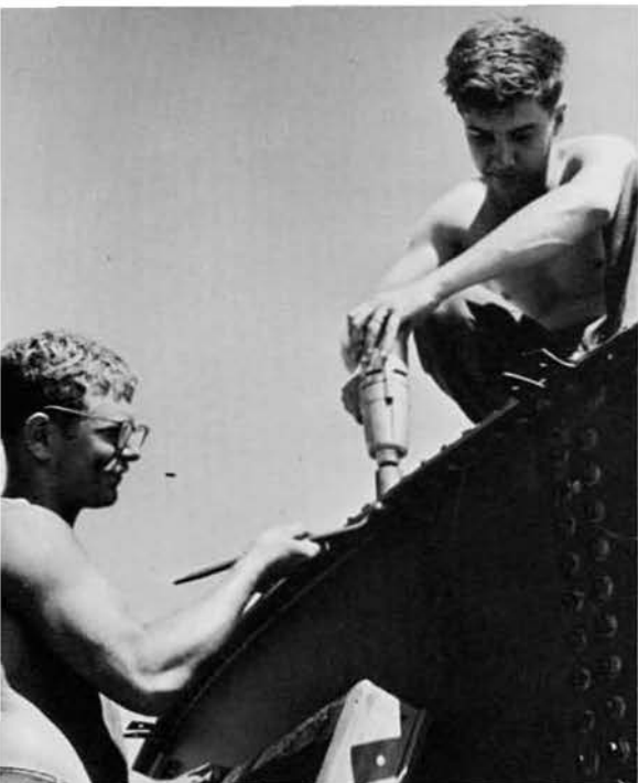
Pendolphina and Dawson finish one of the several tanks done by Charlie Company SW's
