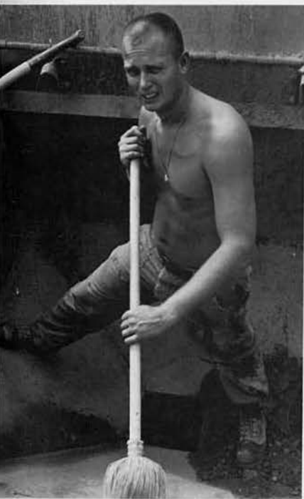
Repovich at the Concrete Batch Plant. Squad Leader Johnson was in charge with Repovich as his assistant throughout the deployment.
