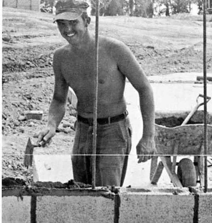
Twenty-foot concrete block fire walls separate the duplex units. BUCN GILBERT stacks them straight.
