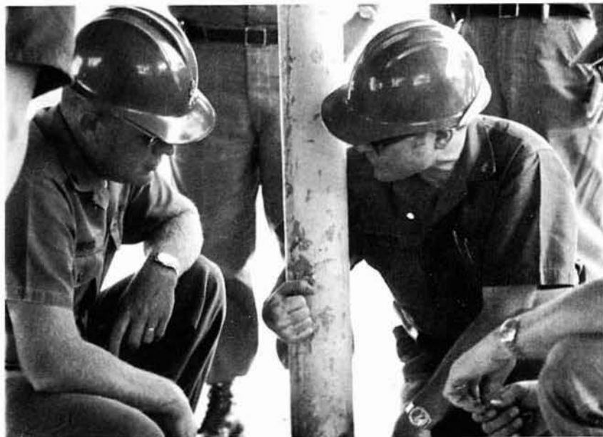
CDR CONNOR (center) offers technical advice to UTC TOMOVICK on welding sleeves for the house columns.
