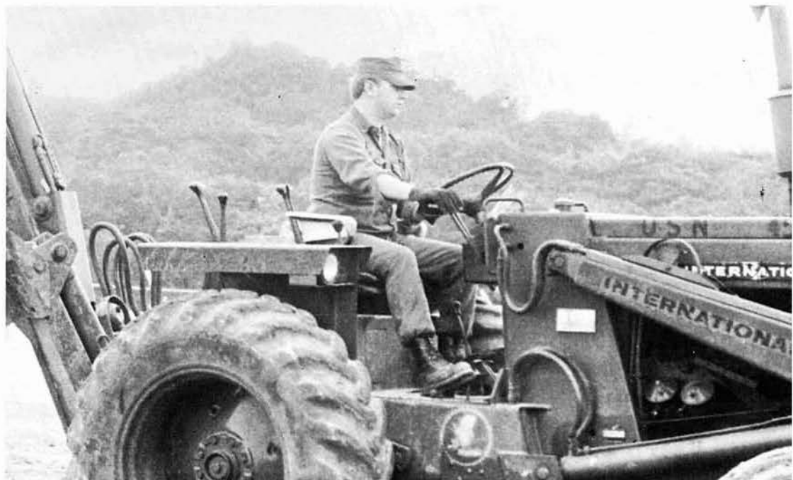
EO3 LEAVITT maneuvers the versatile International Front End Loader. (Left) Directing the equipment loading aboard the LST for Detail KIWI I are LTJG FORTSON and EOCS BENDZLOWICZ.
