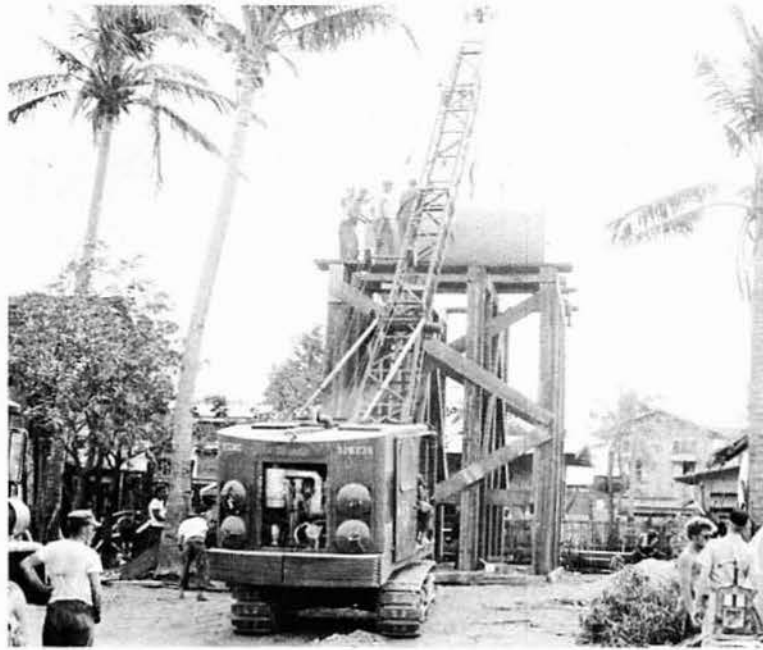
A new water tower for Mindoro thanks to the Seabees and Marines
