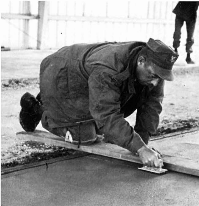
MCAS Futema project crew leader BU1 GROMER gets in the action while preparing a maintenance building floor.
