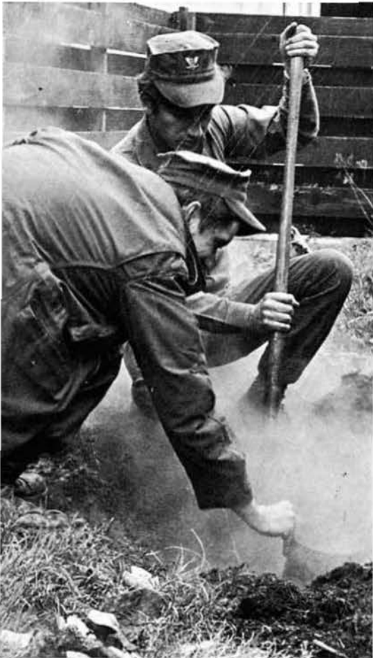
Detail KIWI III Utilitiesmen KOVARIK and FARRIS work to repair a broken steam line at Yokosuka, Japan.
