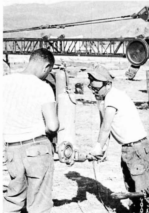
SW1 BROWN and UT2 LODEN thread pipe for use in supporting the water tank.
