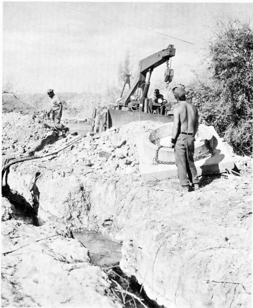
Man hole placement begins for the sewage line project at Officers Beach, Barbers Point.
