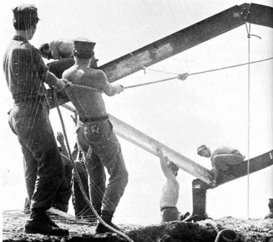
Bravo Steelworkers team up to erect the framework for the new Junior BOQ at Camp Shields.
