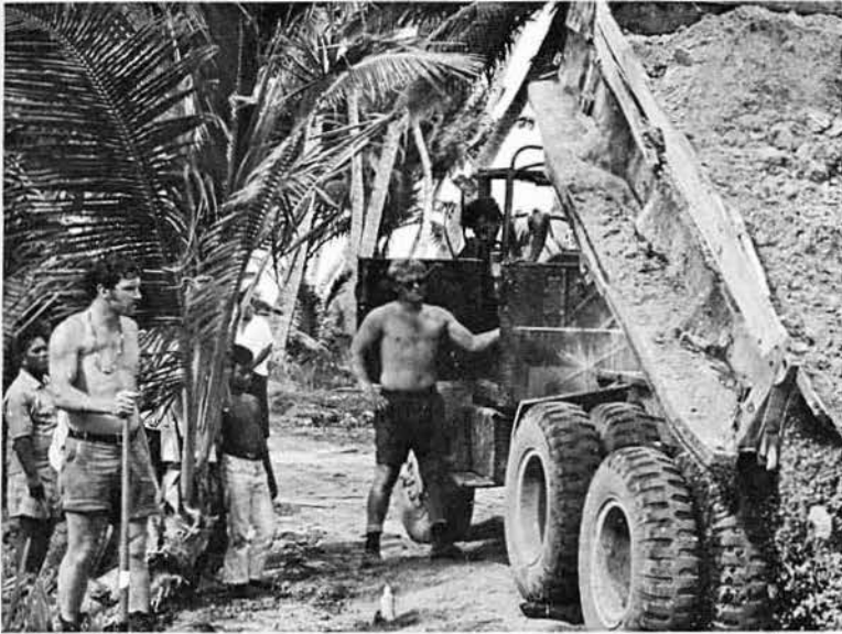
EO's NORK and RENTZ pour dirt for the perimeter road at Moen, Truk Island.
