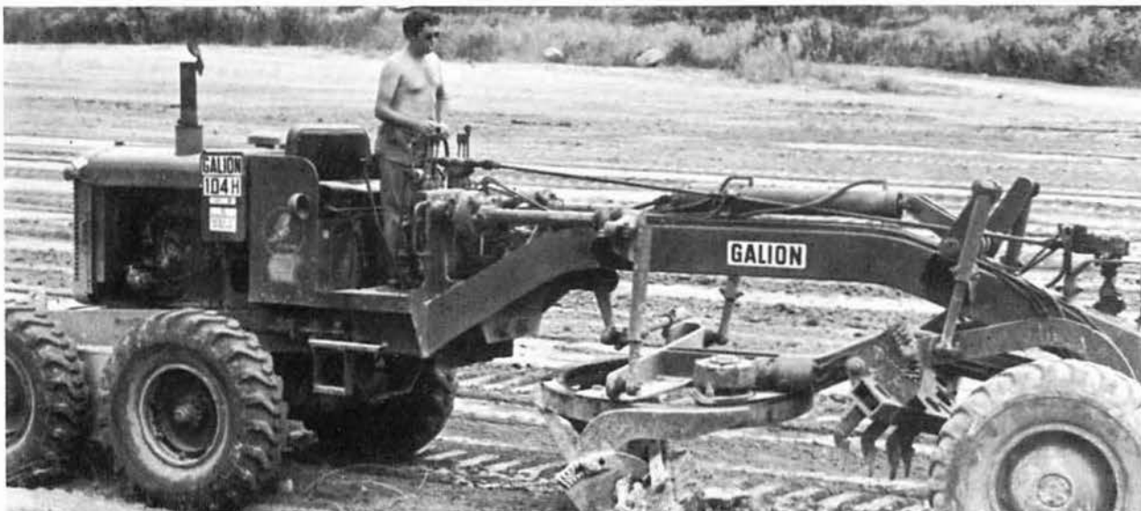
Initial grading on the P-3 rinse rack project for NAS Cubi Point
