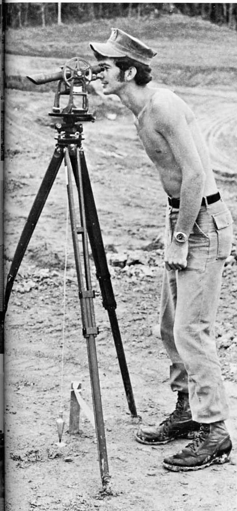
EA3 MERRITT employs a builder's level to shoot forms for the housing pads.
