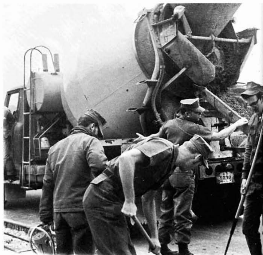
The construction of a driveway for bulldozers was an important addition to the Alfa Company yard.
