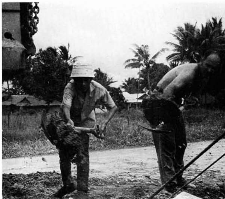
Mixing concrete for village improvements are EO1 WEBB and a Vietnamese youth.
