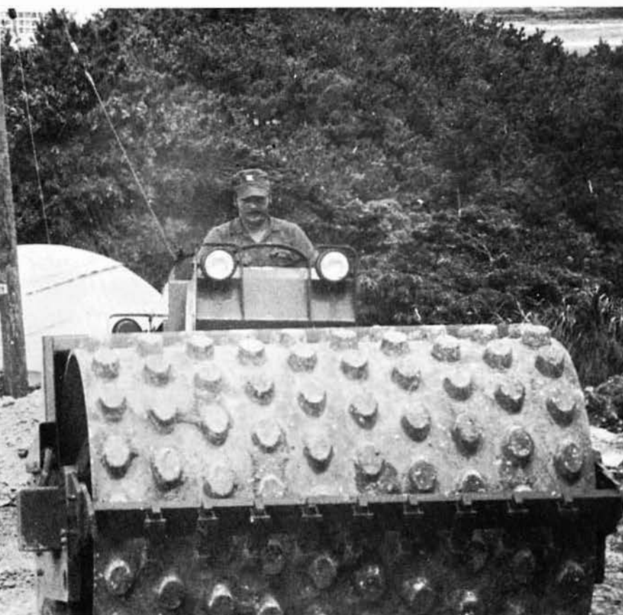
A sheep's foot roller crushes and packs its way while preparing the O-Club roadway.
