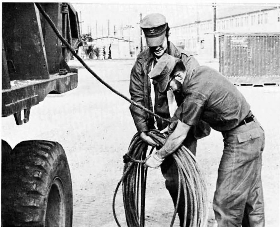
Wire rope is loaded for transportation to the BOQ work site by EO3 RUGGIERO and SW1 INGRAM.
