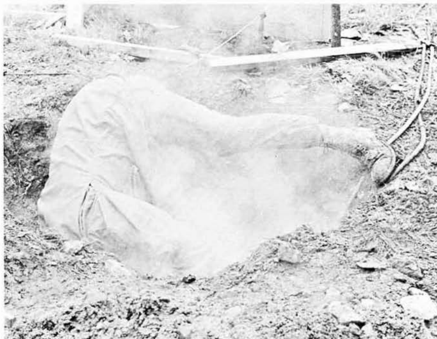
An unidentified NMCB-133 Seabee just plain gets at it while solving a steam line problem.
