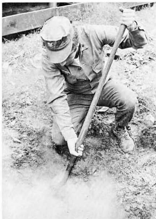
UT3 FARRIS takes care of business on a steam leak.
