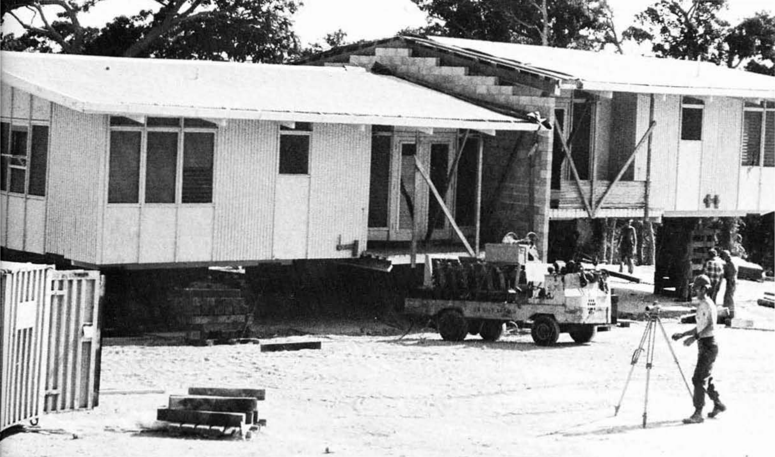
After being relocated to the housing pads, the duplex units were jacked up seven feet for column placement.
