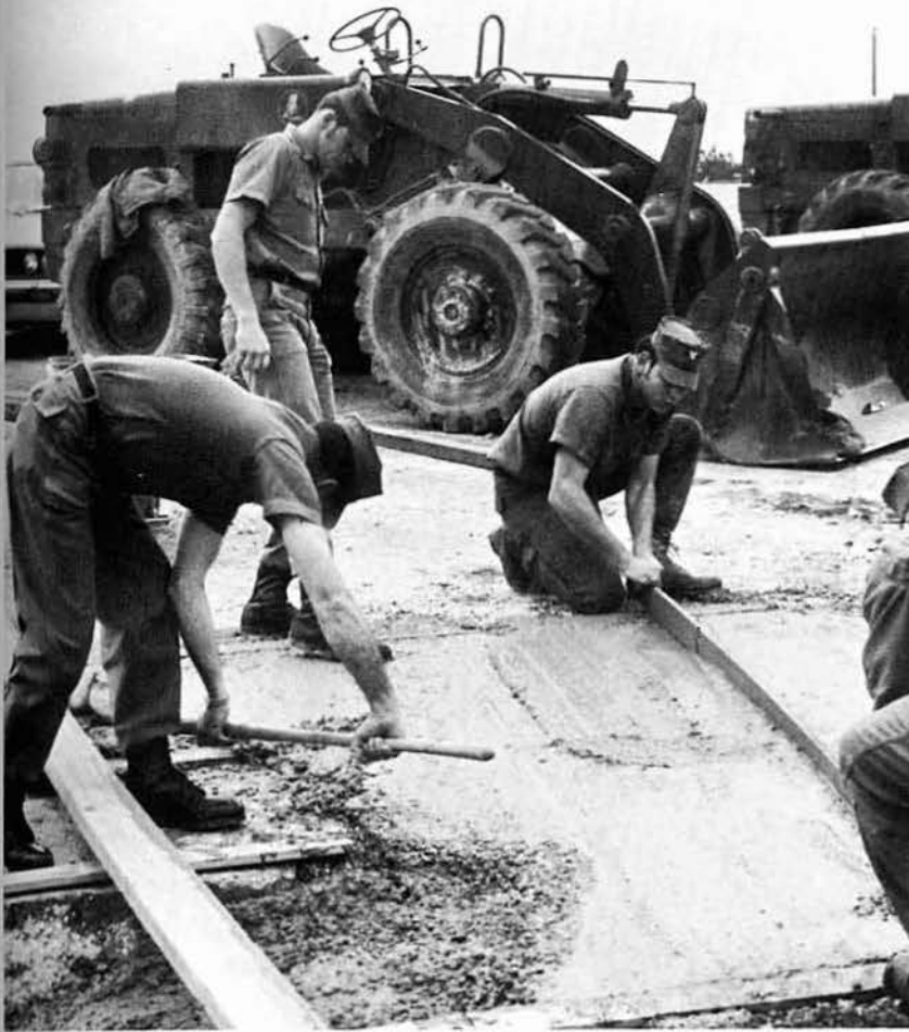
Initial screeding of concrete for the company yard's equipment driveway is done by EQ's CUPP, AHRENS, and CARTMILL.
