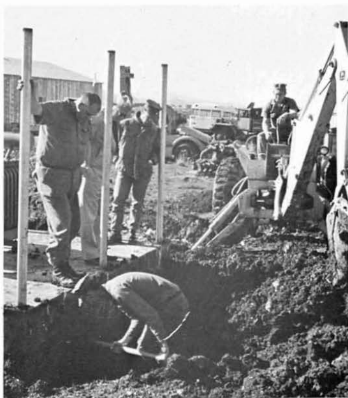
LOOKING FOR THE MISSING CONDUIT.
