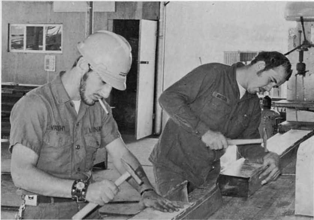
BRAVO SW'S MAKE THEIR OWN DUCTWORK.
