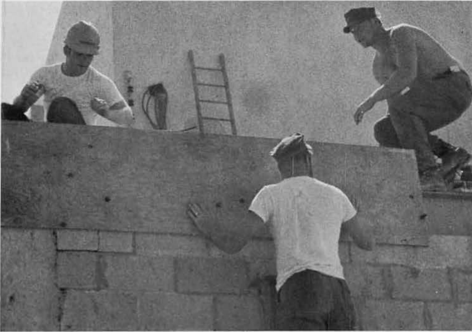
EUCA PITCHFORD, BUCN VAUGHN AND BUCN BLAKEMAN FORM THE LOCKER ROOM ROOF.
