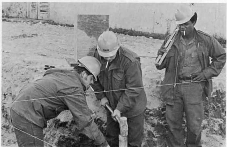
BU2 BREEDEN, CN BROWN, AND CA POWELL STAKE OUT THE LOCKER ROOM ADDITION.
