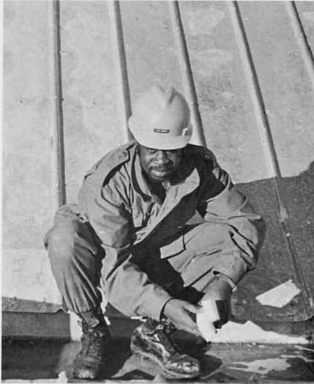
CA BOND FIXING ONE OF THE MANY LEAKS THAT WE FOUND AT THE JET SHOP.
