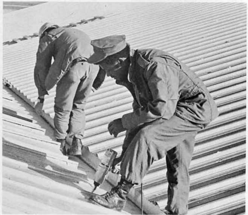
MORE LEAKS TO REPAIR AT THE JET SHOP.
