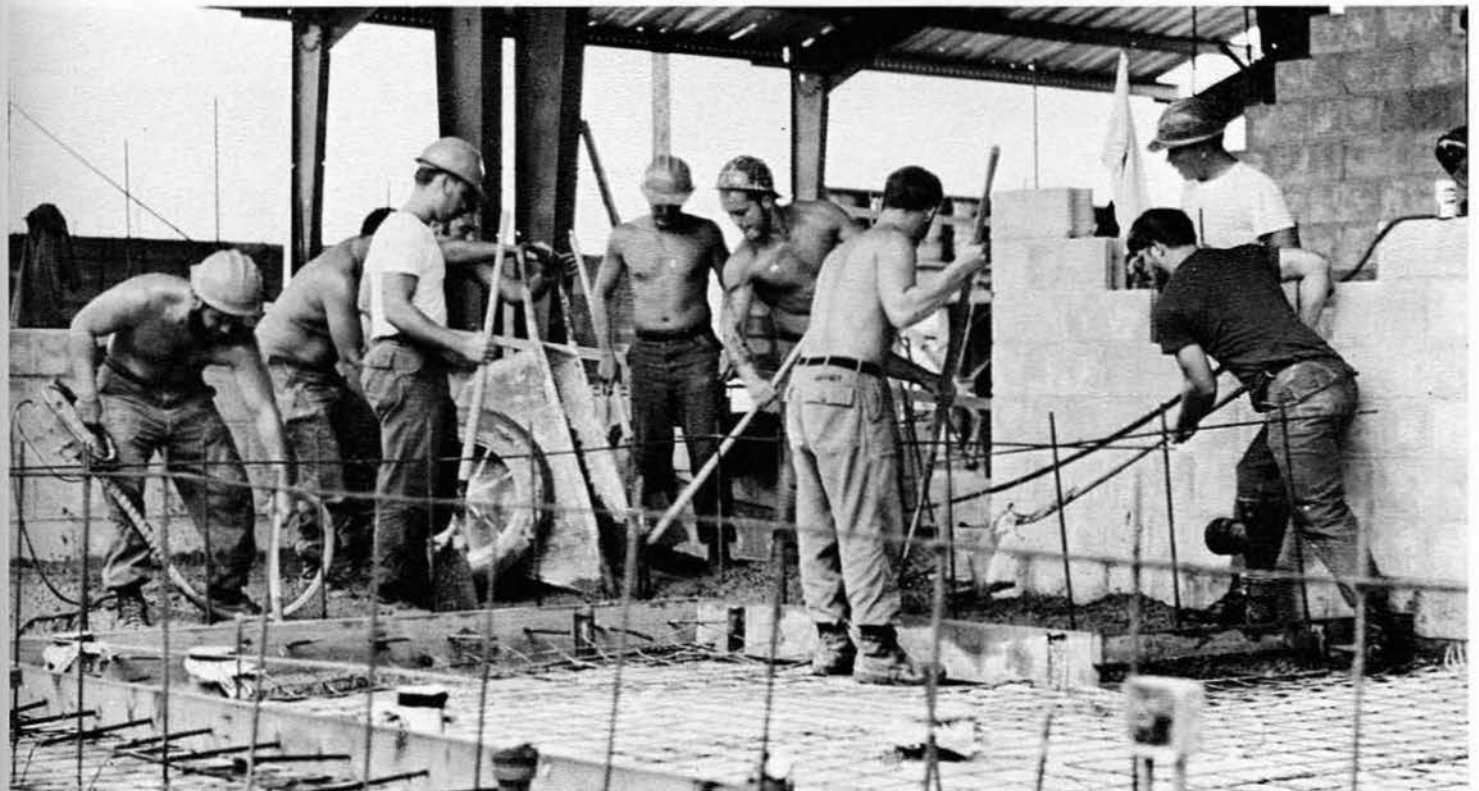
The EM Club crew pouring one of the slab sections for the deck.
