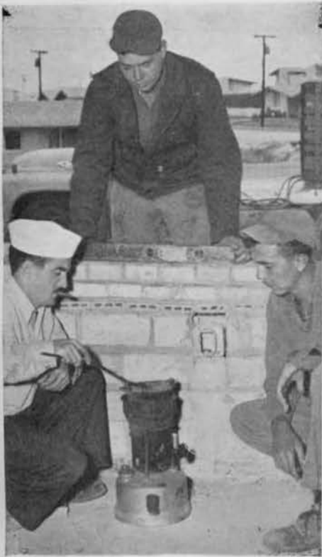
Plumbing at the Gym.
