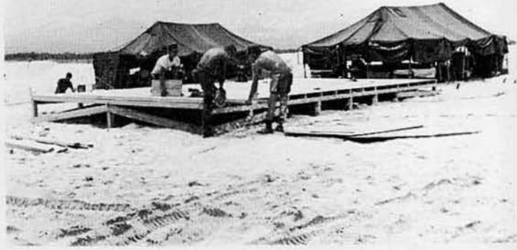
HOI AN IMPROVEMENT --Once barren except for leaky tents housing Marines of the First Battalion, 1st Marine Division, Seabees of MCB-6 finish the floor of this "tinned hut" which will replace one of the tents in the foreground.
