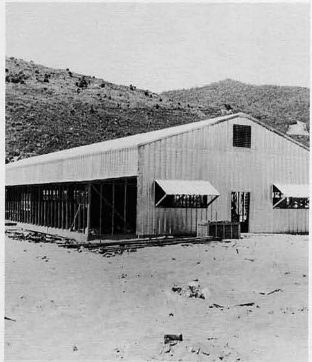
VIEW OF PARTIALLY CONSTRUCTED GALLEY AT TIEN-SHA . WORK IS BEING DONE BY 'C' CO.
