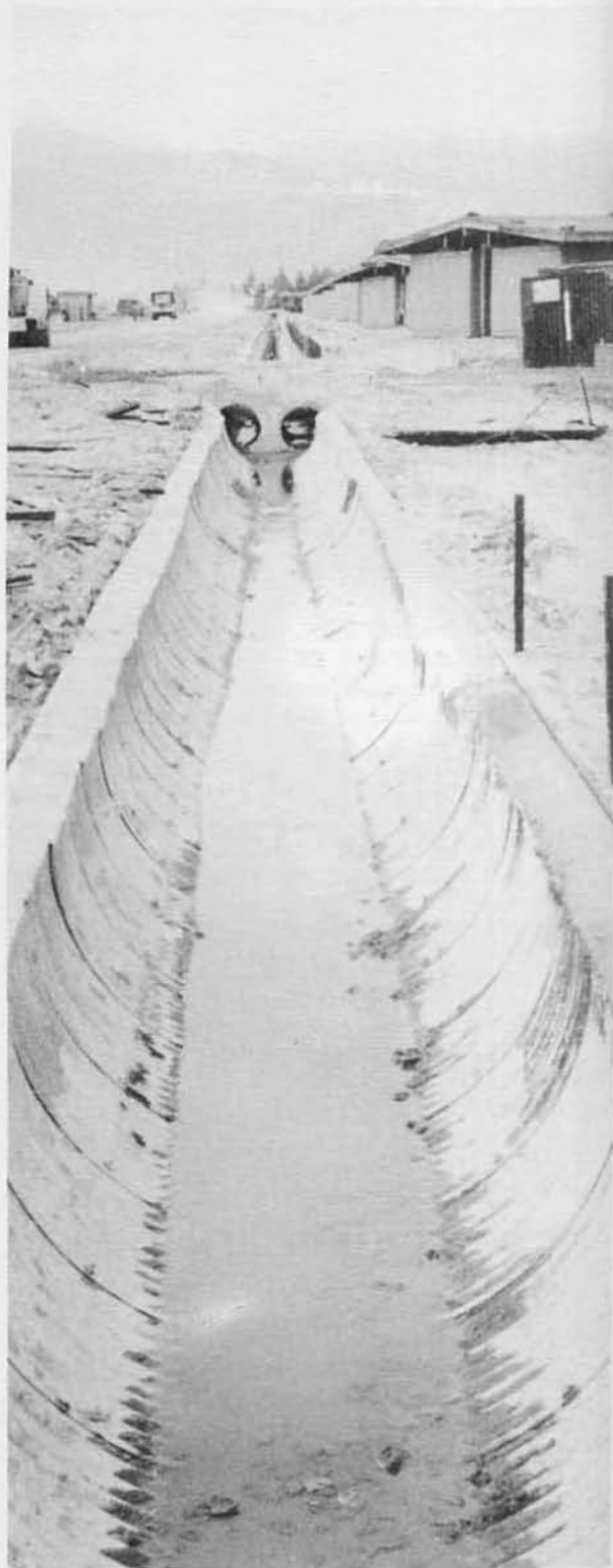
VIEW OF COMPLETED HALF SECTION OF 48" CM.P DRAINAGE DITCH WITH CONCRETE CURB AT COVERED STORAGE.
