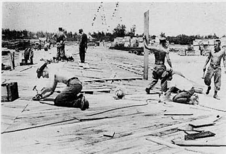
COMBINATION ACHIEVEMENT —The "cold storage" was built by workmen from three MCB-6 companies, A-B-C. Workmen here are busy putting the final touches on the roof of a section of the new facility.
