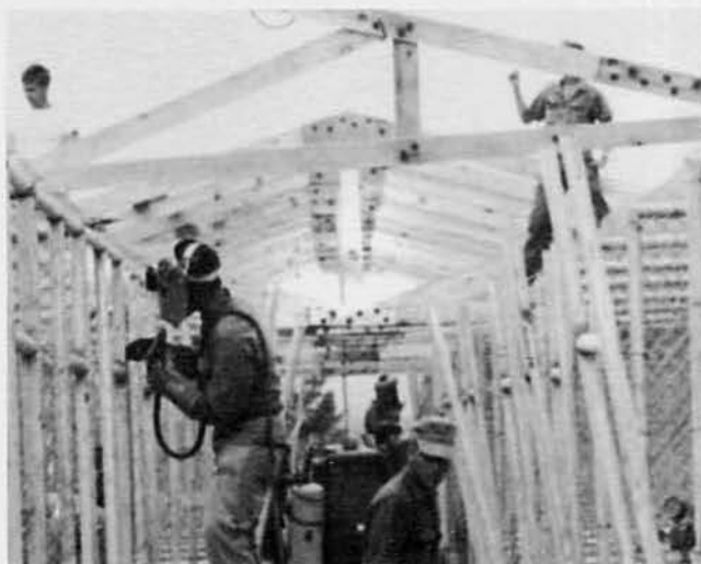
D CO. AT WORK SETTING TRUSSES IN PLACE AT DOG KENNELS - STEEL WORKERS ERECTING CAGES.
