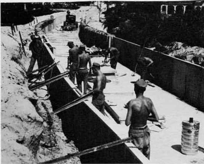
C CO AT WORK SETTING WALL FORMS ON DRAINAGE DITCH AT COVERED STORAGE. NOTE USE OF POST & WIRE MESH IN PLACE OF REBAR.
