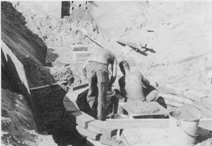
C CO PLACING BLOCK FOR CESSPOOL WHICH WILL SERVE THE HEAD FOR THE ADMIN. AREA AT COVERED STORAGE
