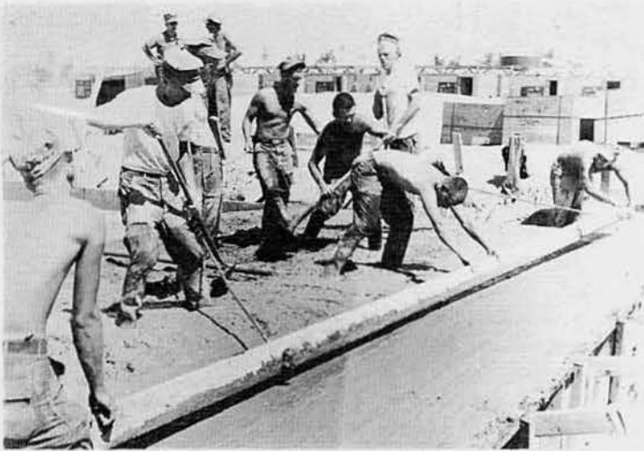
MIXING CONCRETE --This group of MCB-6 Seabees wade in concrete while preparing a base for "reefer pads" outside Da Nang.
