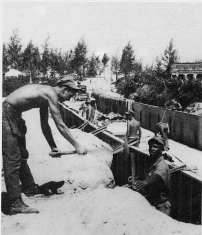
C CO SETTING FORMS FOR WALLS OF DRAINAGE DITCH AT COVERED STORAGE
