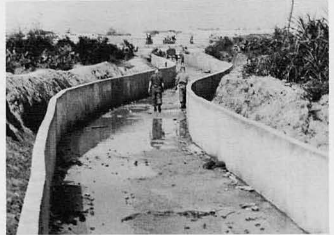
VIEW AT MIDPOINT OF 2700 FT. DRAINAGE DITCH AT COVERED STORAGE. THE DITCH IS 4 FT. HIGH AND 12 FT. WIDE.
