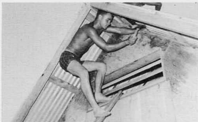
"I'LL FIX THAT LEAK".
