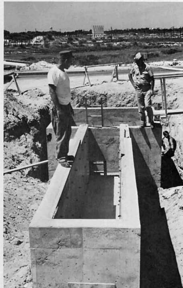
BUI Korpi and Chief Navin inspect the lift station
