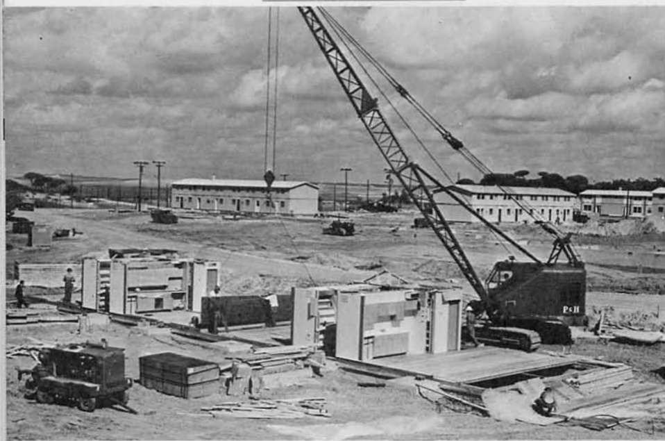
At the height of the deployment, crews could assemble 1.7 units a day.
