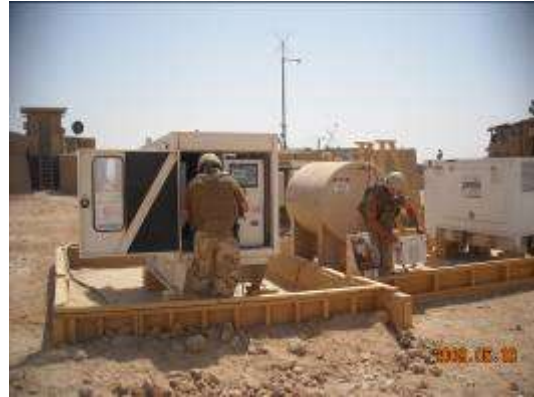
New Generator with spill containment
