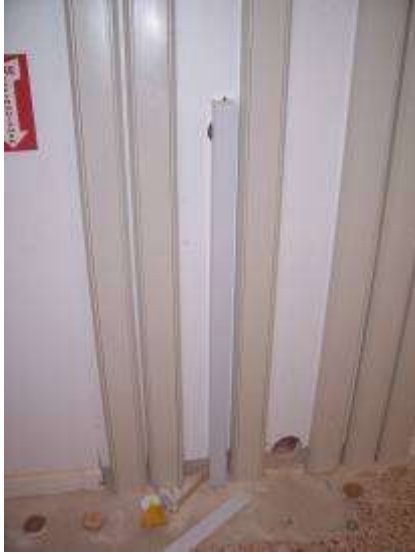
Cable raceways installed
