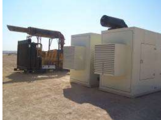
New generator installed
