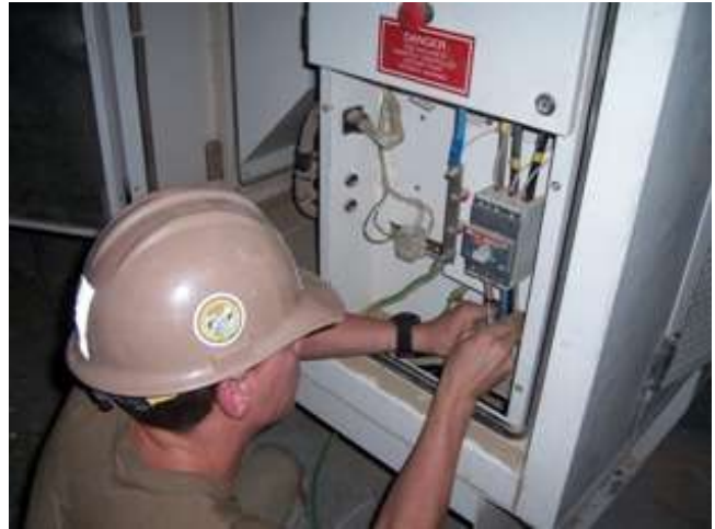
A properly-sized breaker is installed
