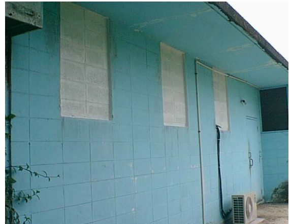
Above: CMU complete in windows and A/C pad and installation complete for Police Station Evidence Room Upgrade.
