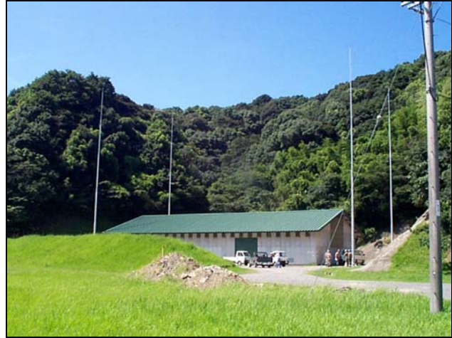
Left, excavation and reinforcing steel placement for lightning mast's concrete foundation. Below, completed steel lightning masts.
