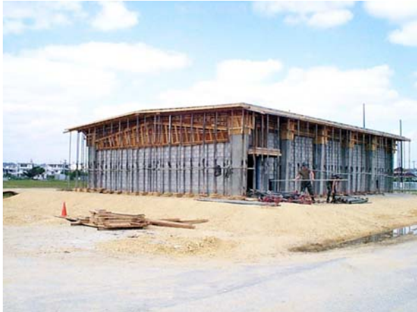
At left, removing screw-jacks after overhead concrete pour. Below, finishing exterior painting.
