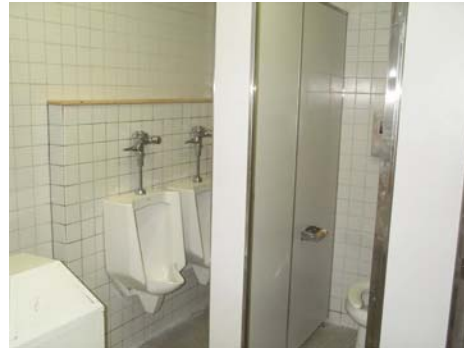
Above: Relocated urinals, commodes and sinks to provide a little more elbow room for the users.
