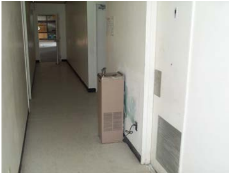
Above: Installed a needed drinking fountain in the new office space and repainted all interior space.
