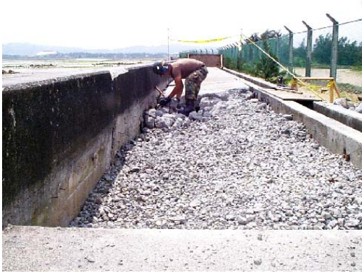
At left, preparing two sections of sidewalk along fenceline for concrete pour. Below, barbed wire along fenceline installed.
