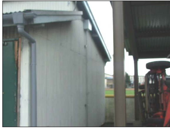
New electrical run to Bldg 47 added power to a storage shed for MWR
