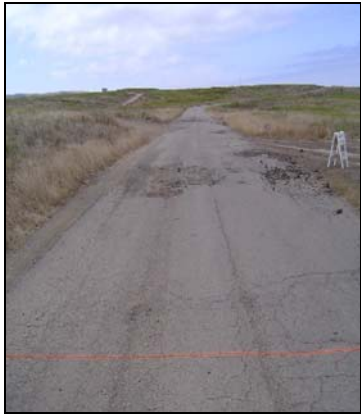
Section one of Ridge Road Repair. 300 lf (before)
