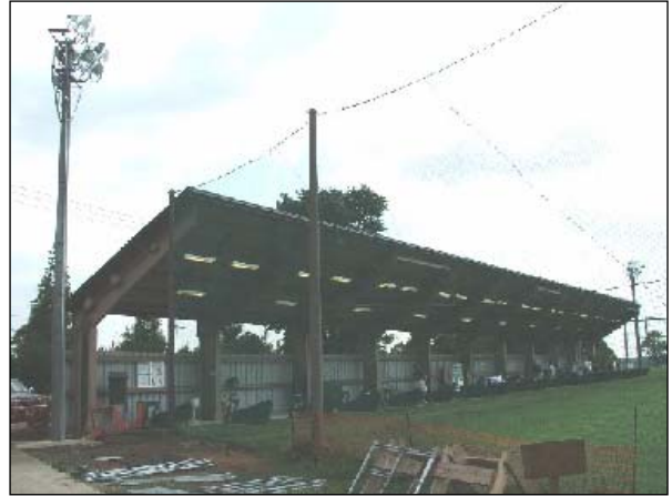
LEFT: CECA Aguila and CE2 Marcewicz installing lights on the new poles. BOTTOM: The project was completed on 16 SEP 05.
