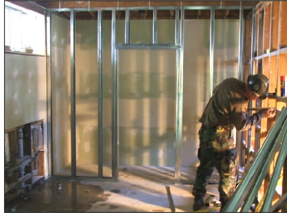
LEFT: Demolition in progress. BOTTOM: UT2 Mayhugh installs new pipes in the bathrooms.
