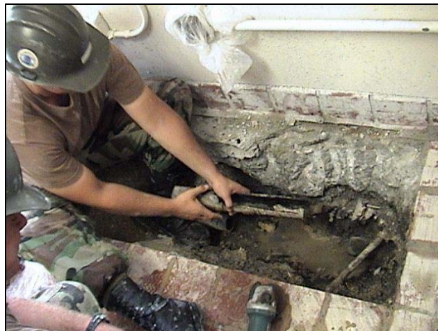
Camp Maintenance crew member retrieves the broken pipe while repairing the Wardroom Galley Drain
