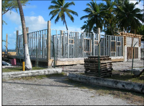
LEFT: Crew finishing pad of sail storage room in new Marina building.. BOTTOM: Front view of Marina site with metal stud walls and partial completion of CMU block at sail storage room.
