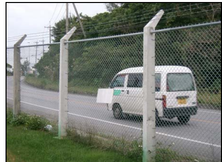
Completed Camp Shields fence repair. Repairs were required after a car accident outside the gate damaged the fence
