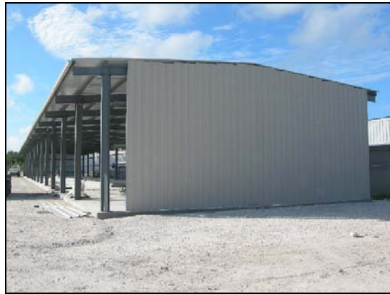
LEFT: Crew placing concrete for concrete footers. BOTTOM: Side view of PEB with partially completed roof sheathing.
