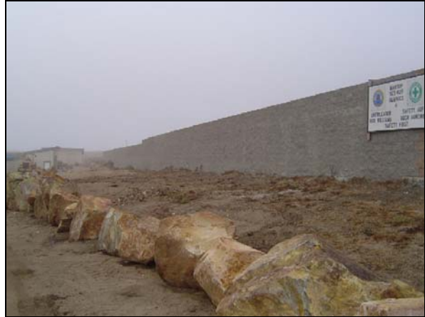
LEFT: Block wall prior to commencement of work. BOTTOM: Completion of wall.
