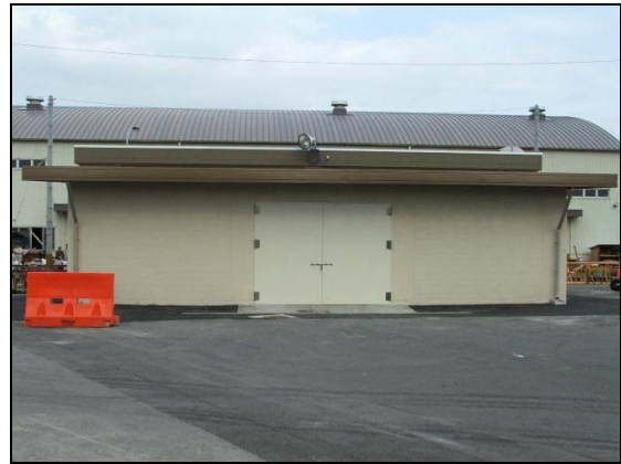
LEFT: Project was taken over at 50% complete with CMU block walls in place. BOTTOM: The completed project.
