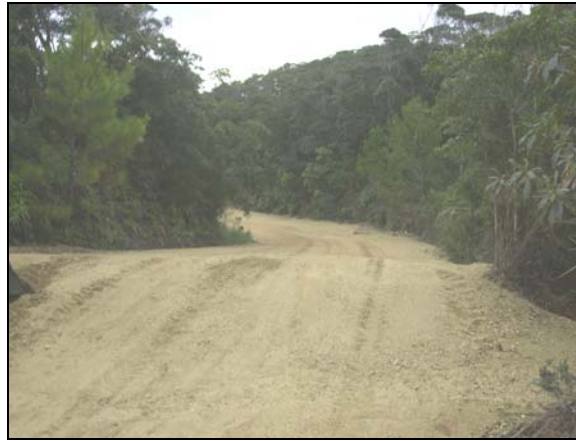
LEFT: The road prior to repairs. BOTTOM: Completed project including diversion ditches and soil stabilization.
