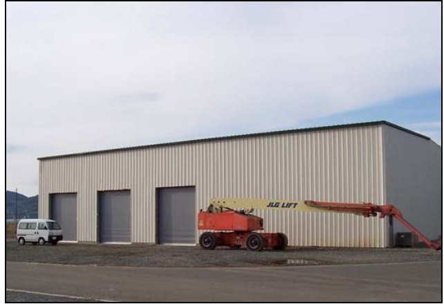
LEFT: BUCN Shonewetter helps install roof insulation and panels using a manlift. BOTTOM: Completed Sakibe Fire Station.
