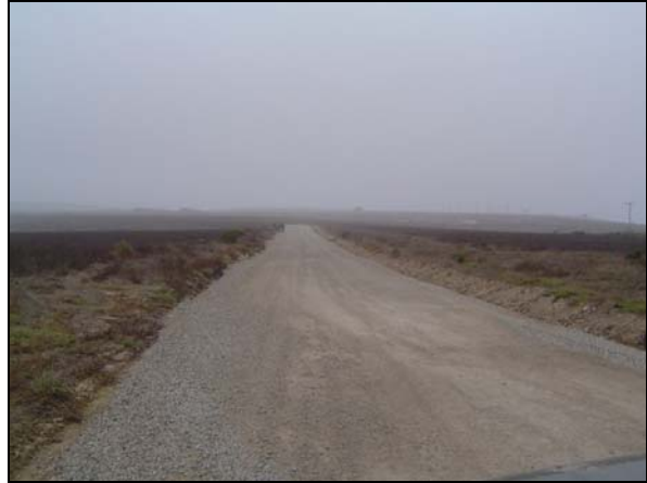
LEFT: Dozer placing sub base course down at beginning of phase. BOTTOM: Section of AVMR completed.
