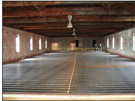
LEFT: Crewmembers BU3 Audie, BU3 Greenert, and SW3 Jacques guide one of fourteen columns in place. BOTTOM: Completed mezzanine decking for the 2 nd floor of the warehouse.
