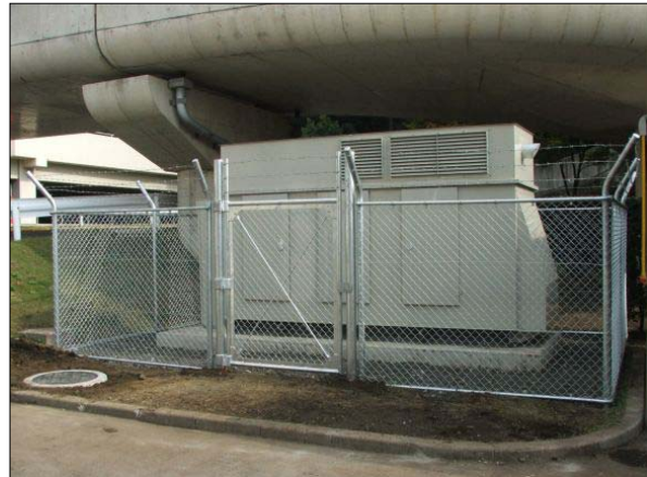
LEFT: Completed concrete pad. BOTTOM: Completed installation of concrete pad, generator and fencing.
