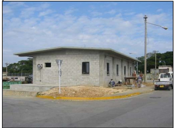
LEFT: Crew placing the concrete slab. BOTTOM: Crew is installing windows doors and interior finishes while the exterior area is prepared for paint.
