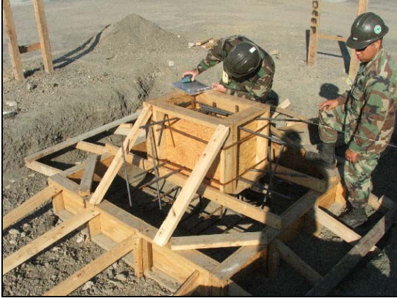
LEFT: QC, BU1 Fiser, checks clearances in one of twenty-four footers while the Project Supervisor, BU2 Celaya looks on.
