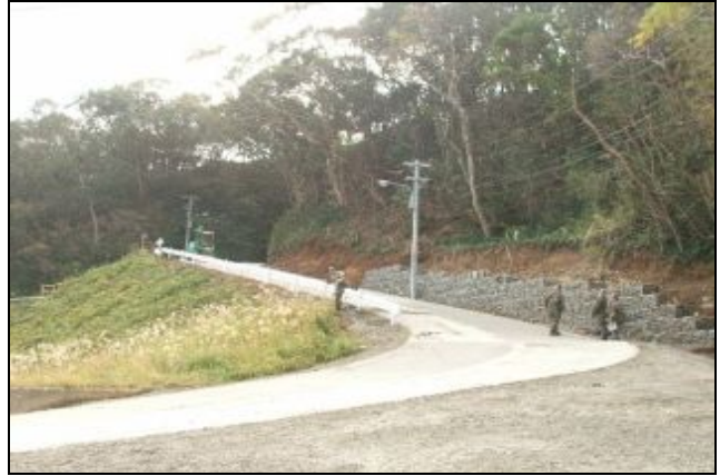
LEFT: Yokose crew works to place concrete for the upper section of roadway. BOTTOM: Completed roadway.
