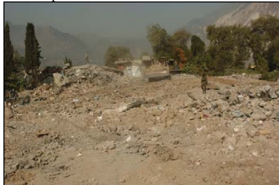
LEFT: Air Detachment Equipment Operator clears debris of Muzaffarabad University. BOTTOM: Muzaffarabad University debris clearing near completion.
