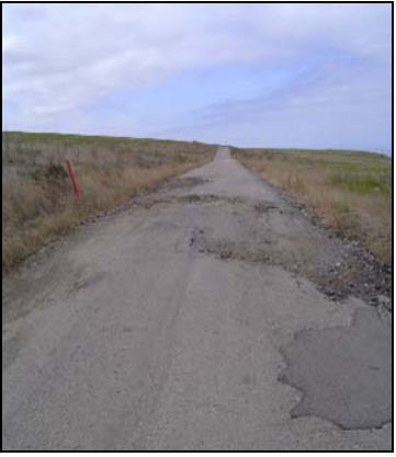
Section Two of Ridge Road Repair. 167 lf (before)
