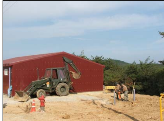
LEFT: Block walls being installed on 11 October BOTTOM: Building at 80% complete as of 22 November.
