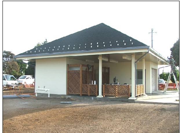
LEFT: The heavy timbers and steel beams of the roof structure are all in place. BOTTOM: BU2 Melendez puts the finishing touches on the fascia board.
