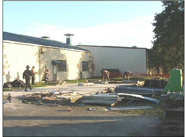
LEFT: Building 585 before the start of work. BOTTOM: The project crew finishes demolition of the existing building.
