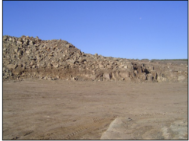
LEFT: Early stage of Mid-Island Quarry development. BOTTOM: Continued development of the Mid-Island Quarry.
