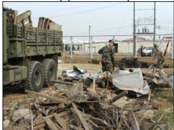
Seabees removed a sizeable pile of debris that was remaining from previous the year's typhoon destruction.
