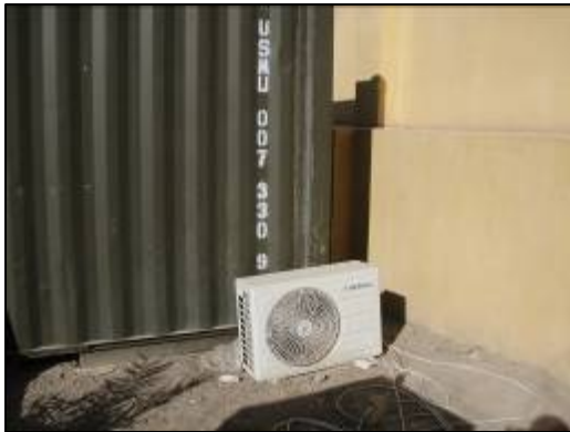
Installed A/C unit.
