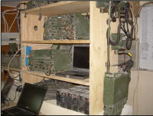
Fig. 22 – Communications and data networks in Ar Ramadi.
