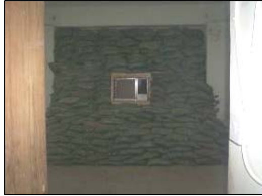
Installed A/C unit.
