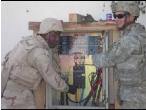
Electrical upgrade trenching operations.
