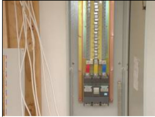
Installed electrical panel by the contractor.
