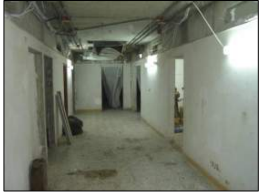
Lighting installed in the main facility.
