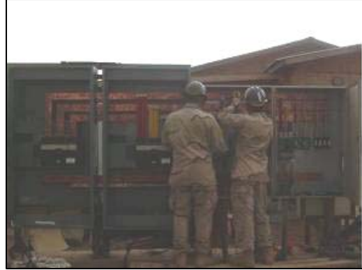
Electrical panel and bus installation.
