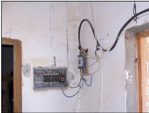
Original Electrical at COP OK Corral.
