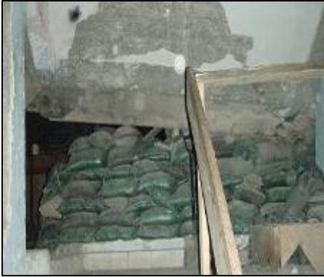
Structural failure at OP Horea. Member being held up by sandbags.
