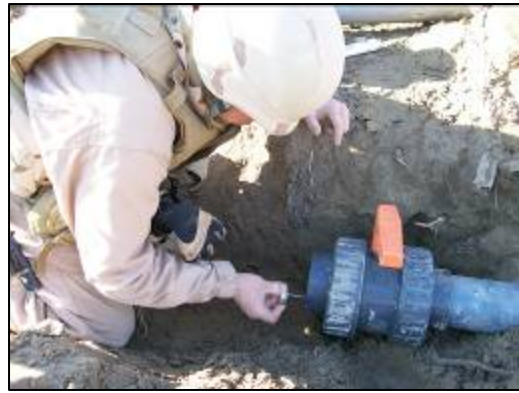
Gluing a joint on a valve prior to completing the pipe connection.
