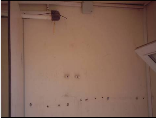
Missing water heater.
