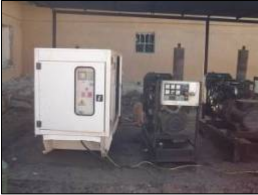
Completed installation of the new generator located next to the old generator.
