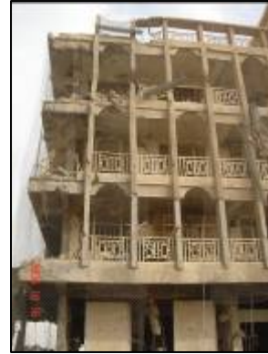
Damage to the structure at OP Hotel. First deck being supported by T-walls.
