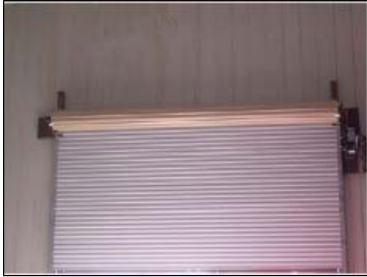
Inside view of roll-up door mechanism.
