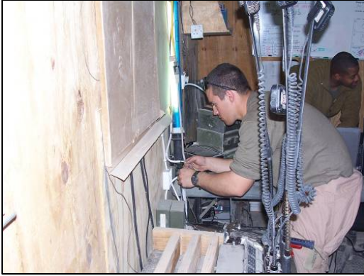
Original Electrical at OP Dunlap.
