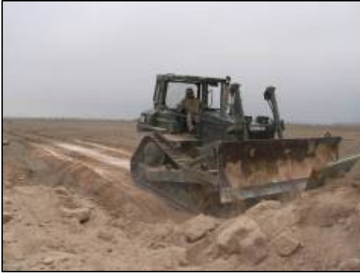
Equipment Operators improve perimeter road berm to cover and conceal runners from Camp Habbaniyah.
