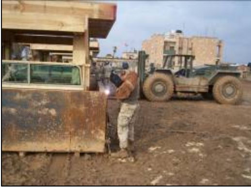
Installation of steel plating on a “Crow’s Nest” in the Delta Co. fabrication yard.
