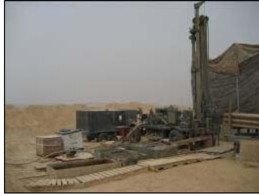
Water Well in operation.
