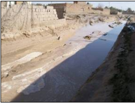
Flooded out Main Street prior to repairs.
