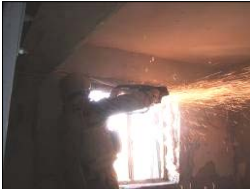
Removal of the bars around a window to allow installation of an A/C unit.
