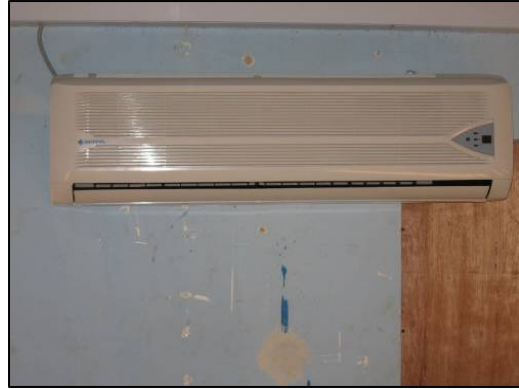
Installed ECU unit in MITT berthing.
