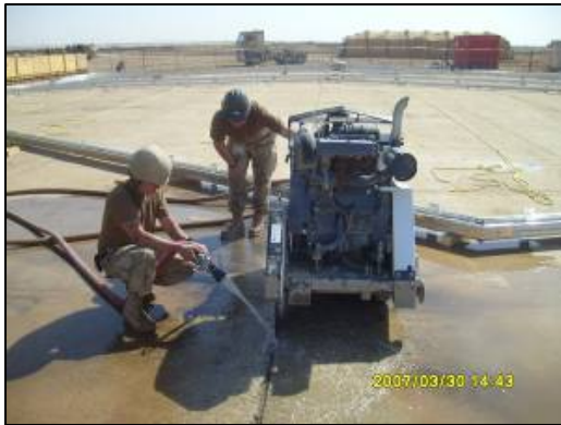
Saw cutting the existing pad in preparation for the steel maintenance pit.
