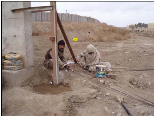
An Iraqi engineer assists with installing of cables for the Habbaniyah ECP.
