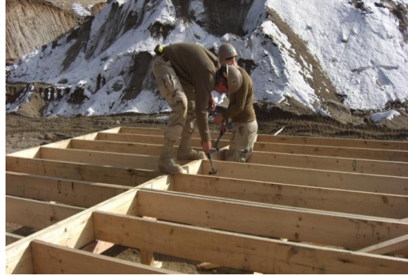
BU2(SCW) Condon and BU3 Richardson positioning the floor joists for a B-Hut.
