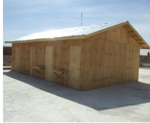
Photo of project site after B- hut was Completed, prior to BOD.
