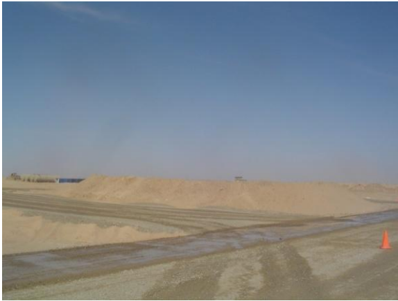
HLZ Fuel Farm with bermed up area and road prepped around fuel farm
