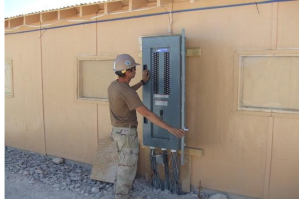
Confirming proper labeling of circuits.
