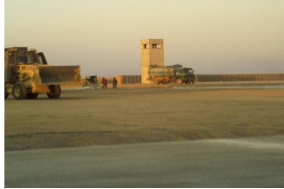
MEP at beginning of construction.
