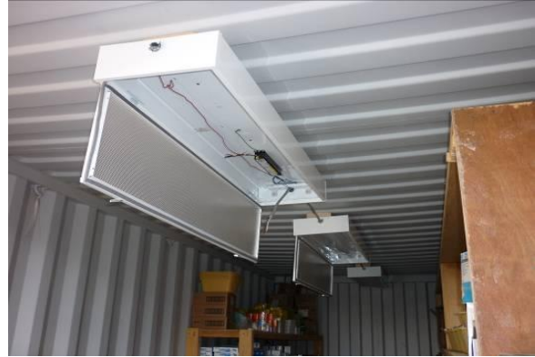
Connex box outfitted with electrical.
