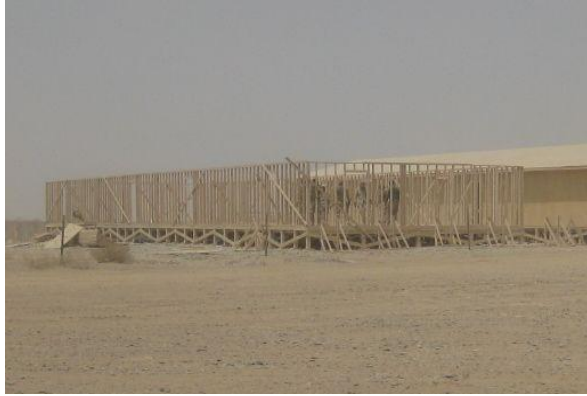
RCT TOC 2 at Turnover
