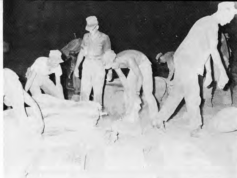
The "Men of TEN" work through the night (above) repairing the Camp Evans runway.
