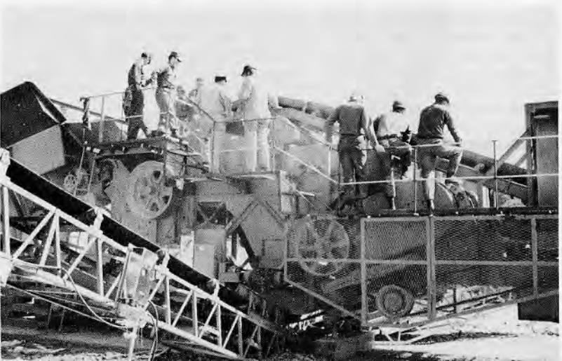
An actual rock crusher installation at Port Hueneme provides the Seabees with on-the-job experience that will be valuable while deployed to Vietnam. This crusher is just one of many project sites located in the Port Hueneme area.
