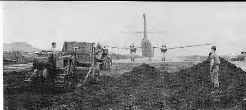
Khe Sanh runway (above) is being upgraded and rebuilt by Seabee Detail BRAVO from CBMU 301 during the days just prior to the enemy siege. The Detail remained at Khe Sanh during the enemy offensive to continue runway and base repairs which were many.
