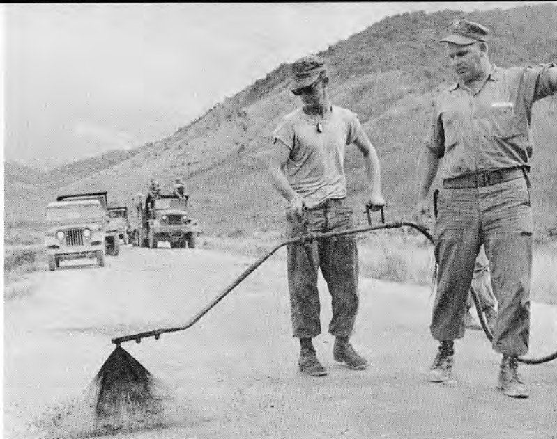
Seabees from NMCB 121 spread oil on the road bed to firm up the surface of National Route One in the photograph above.
