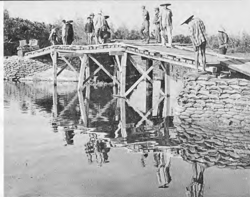
A small bridge built in the Vinh Loc District of Thua Thien.
