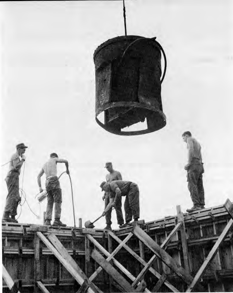
NMCEB 5's Delta Company crew (above) pours concrete into forms on the "Teapot" job site.
