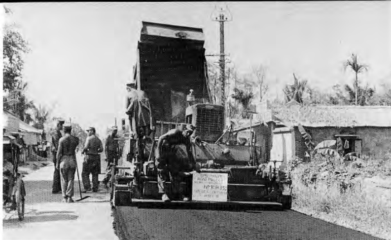
NMCB 133's asphalt spreader applies asphalt to the Col Co Road (above). The Seabees surfaced the roadbed prepared earlier by NMCB's 3 and 8 as denoted by the sign on the spreader.
