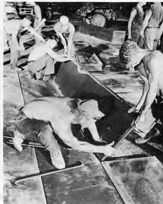
Seabees worked throughout many a night in 1968 to make emergency runway repairs.
