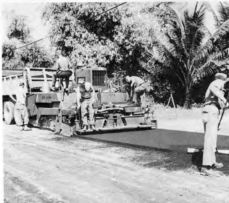
NINE's paving crew place the first lift of asphalt on Route 541 located in the Danang complex of bases, hamlets and a city in the photograph below.
