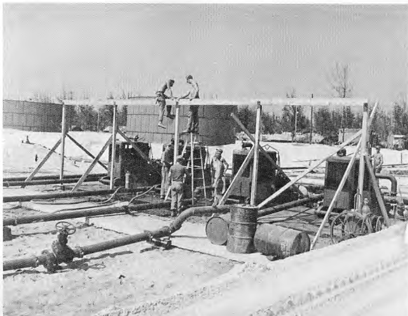
On the right, Seabees make repairs to the Hue Causeway during the monsoon season while in the photograph below, other members of the battalion install a POL pumping station at the Tan My POL Farm on Coleo Island northeast of Hue City.
