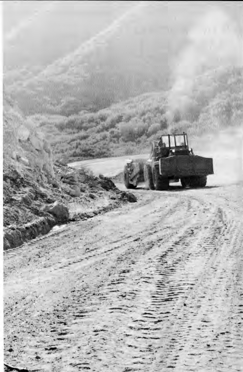
The construction of fire breaks, roads and right-of-ways provides the Seabee equipment operator with excellent on-the-job training while his battalion is homeported at Port Hueneme.
