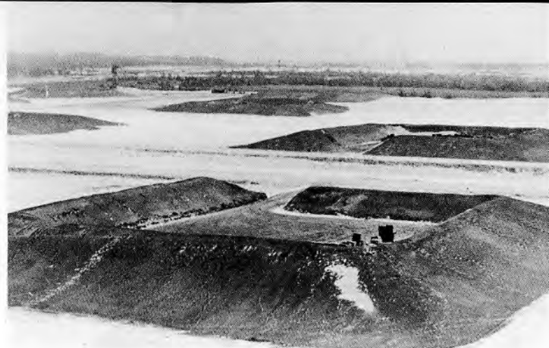
NMCB 6 repaired and constructed 13 Ammunition Supply Points (above) for the Army's Americal Division during its Chu Lai deployment.
