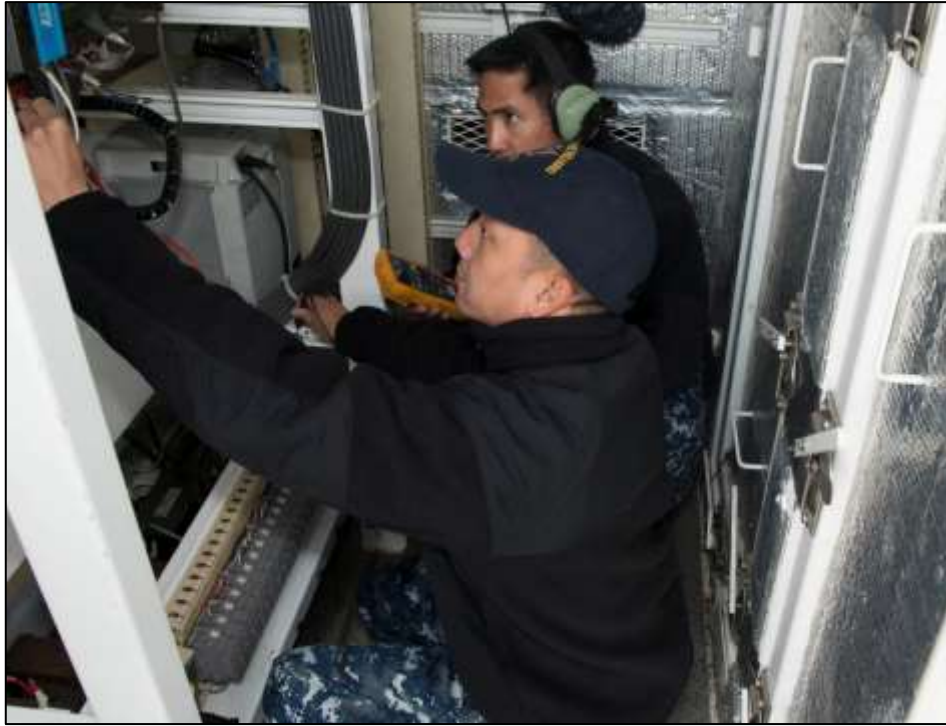
Sailors perform diagnostics on newly installed equipment during CNO Selected Restricted Availability, 2014.
