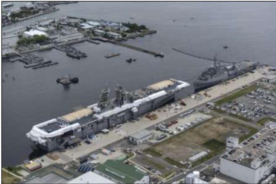
Resurfacing of USS BONHOMME RICHARD's flight deck during CNO Selected Restricted Availability, Sasebo Harbor, 2014.
