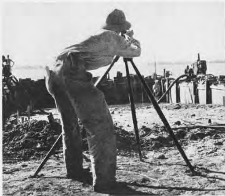
SEAPLANE landing ramp goes up where this Seabee surveyor is laying out cofferdam site
