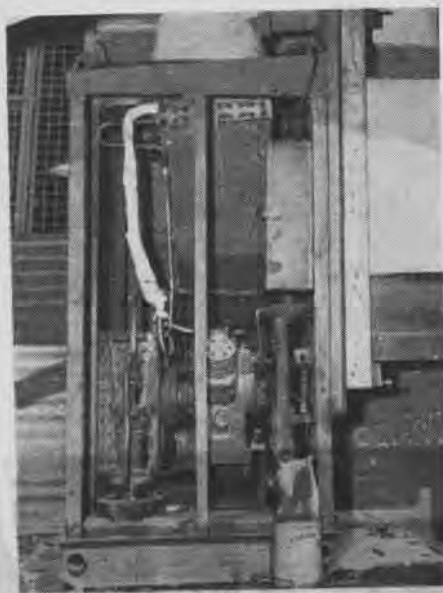
REFRIGERATING UNIT REDUCES HUMIDITY
