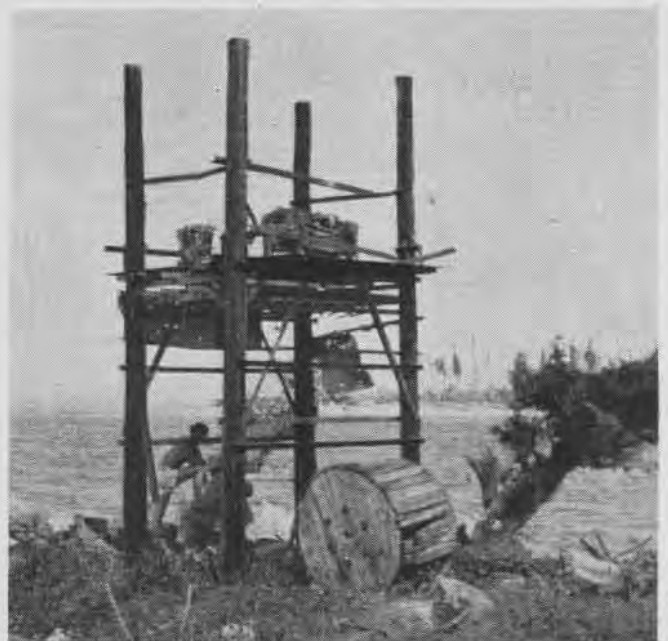
Jap transformer is set on platform near the beach on one of the Marshall islands. This is in plain view for the aerial cameraman
