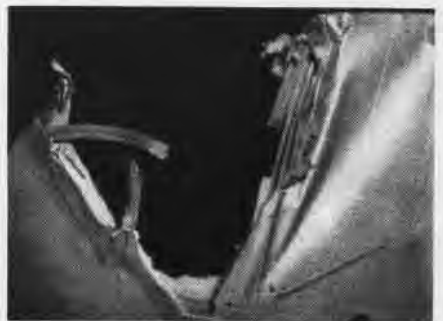
LIGHTNING LEFT WIDE HOLE IN ELEVATOR
