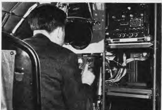
Neptunes carry plenty of radar and radio gear; this picture shows camera installed for photographing traces on scopes
