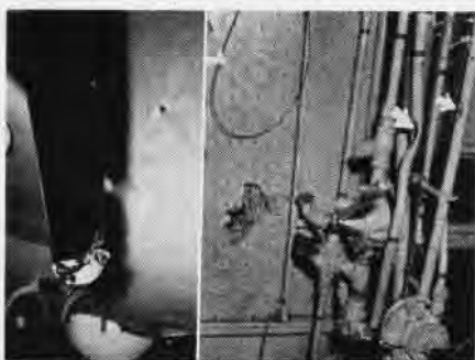
PHOTOS SHOW DAMAGE TO PROP AND FUEL LINE
