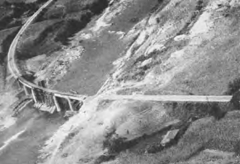
THIS AERIAL photo shows Korean bridge repaired after previous Navy strike, heavy timbers shoring up roadbed, end unfinished
