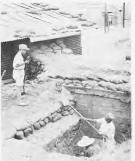
SOUTH Korean laborers dig bomb shelters; sandbags on tin roof are air raid defense
