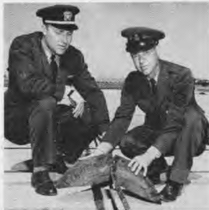
CROSS-DECK pendant support at NAS Miramar is inspected by Ltjg. Mosher and Cobb.
