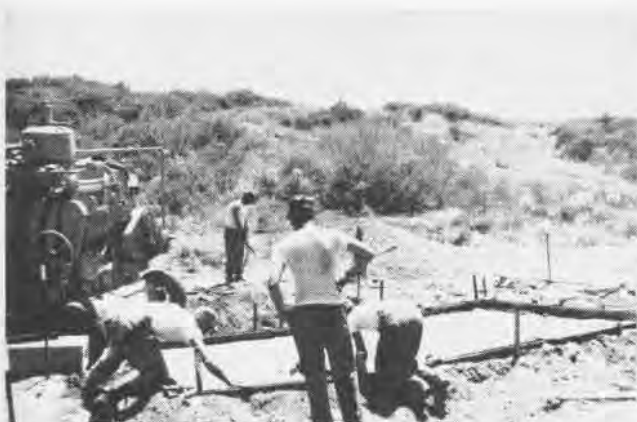
MARINES construct "gallinaceous guzzler" (underground water tank) at Camp Pendleton. Tank provides constant water source for quail.
