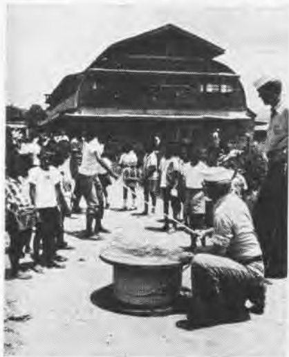
KEARSARGE men with their "helpers" string electric cable before rewiring the classrooms.
