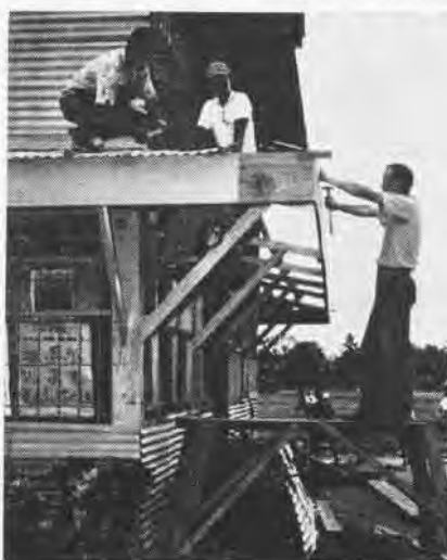
J. A. WILLIS, SH3 (R) , and Philippine co-workers build new rain awning for school.
