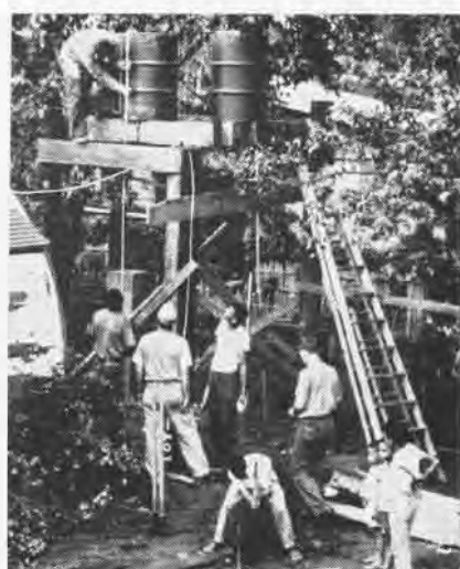
GALLON DRUMS are mounted on specially built platform for new water supply system.
