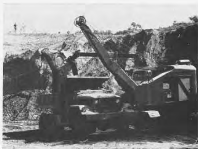
EARTH FILL pours into a waiting dump truck as MCB-10 Seabees work in round-the-clock shifts to get the Chu Lai airfield ready.
