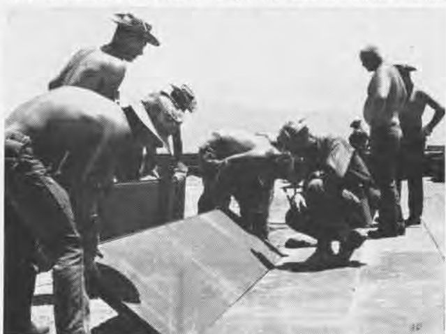
SEABEE CREW eases a 2-by-12 foot aluminum matting section into place on expeditious airfield. Each panel was placed by hand.
