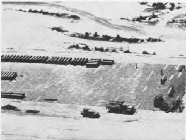
ALUMINUM MATTING is staged at airfield site as MCB-10 crews work on runway. Seabees averaged 400 feet per 8-hour shift.
