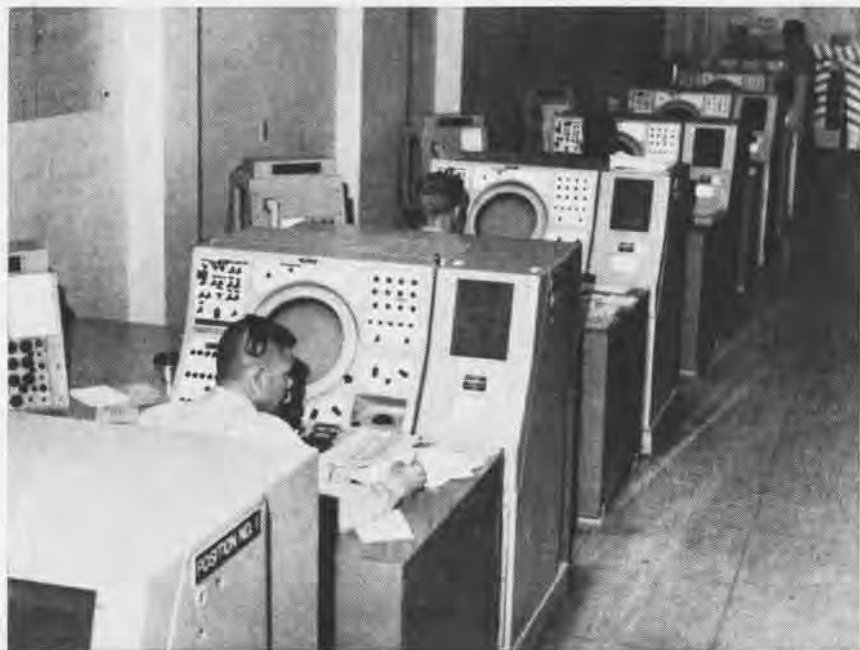
SURVEILLANCE consoles show the positions of all aircraft flying in FACSFac's control area, allowing operators to monitor the situation and re-route traffic if it is necessary.
