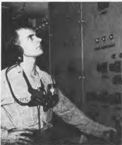
OPERATION of the ship's service electrical switchboard is this man's assignment.
