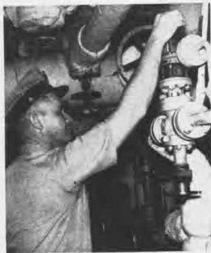
CHIEF aboard USS Intrepid operates steam regulator in one of the carrier's firerooms. ton bombers every minute.
