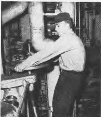
FEED WATER control valve on one of Kitty Hawk's boilers is opened by D. J. Short.
