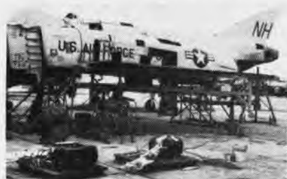
BEGINNING to look like an aircraft again, the Phantom receives obsolete components.
