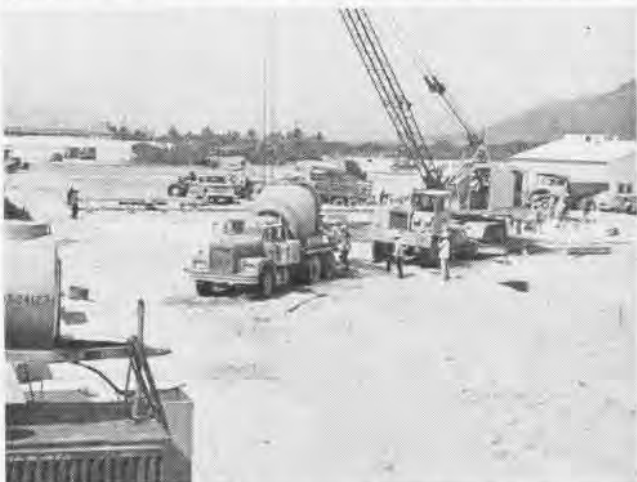
BUILDING barracks, messing facilities and working spaces has meant moving mountains of sand and daily winds are a constant problem.
